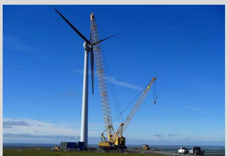
A 900-kilowatt Emergya Wind Technologies turbine began operating in 2019 in St. Mary's, Alaska. The MIRACL project analyzed its resilience benefits and value streams, along with the potential benefits of more advanced control. Photo from DOE
