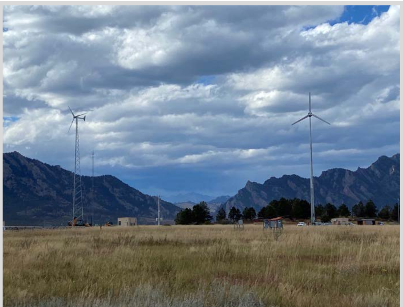
Two of three new distributed wind turbines were installed in September 2023 at NREL's Flatirons Campus. Photo by Ian Baring-Gould, NREL
